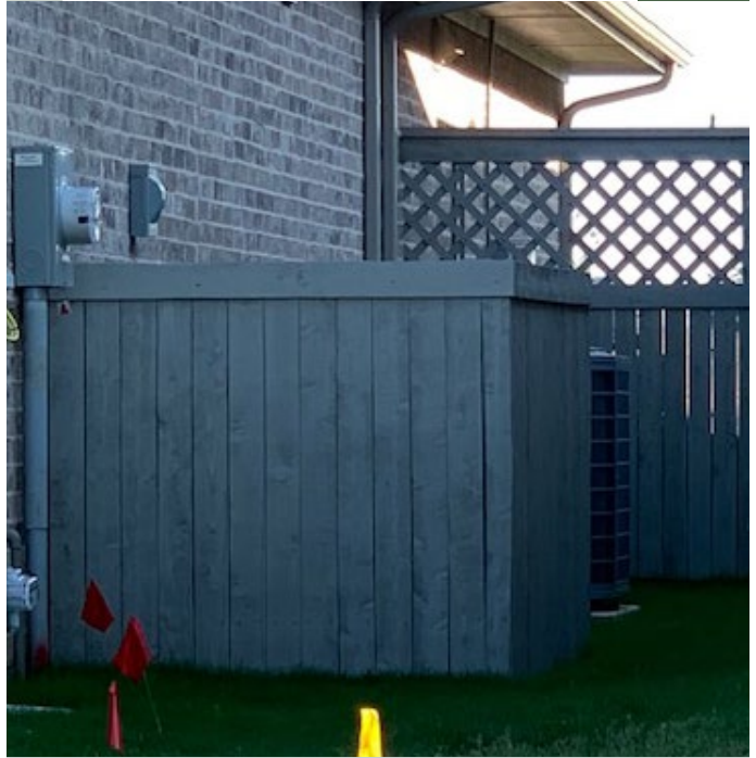
Where home spacing is too tight, a single 4ft tall vertical picket screen may be permitted. The screen should be stained to match the fence.
