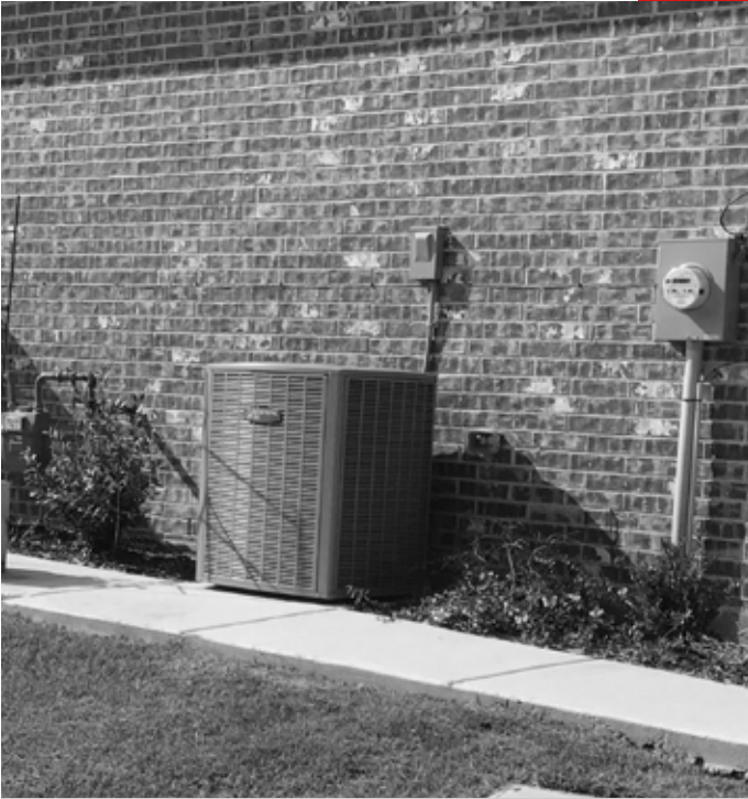
A/C unit must be appropriately screened.
