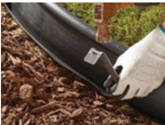
Rolled plastic edging is prohibited.
