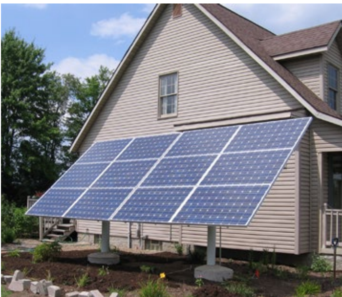
Ground-mounted solar panels are not permitted.
